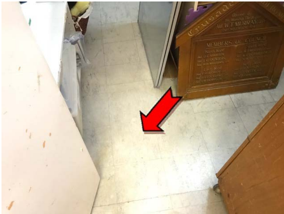
Photo 3. Interior, ground level, southern store room, floor coverings – asbestos-containing vinyl floor tiles.
