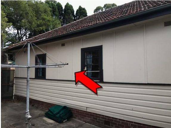
Photo 1. Exterior, throughout, wall paneling – asbestos-containing fibre cement sheeting.
