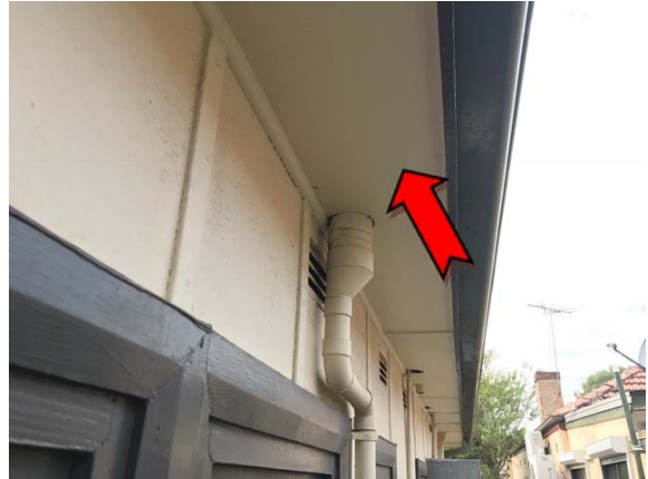
Photo 2. Exterior, throughout, eaves – asbestos-containing fibre cement sheeting.
