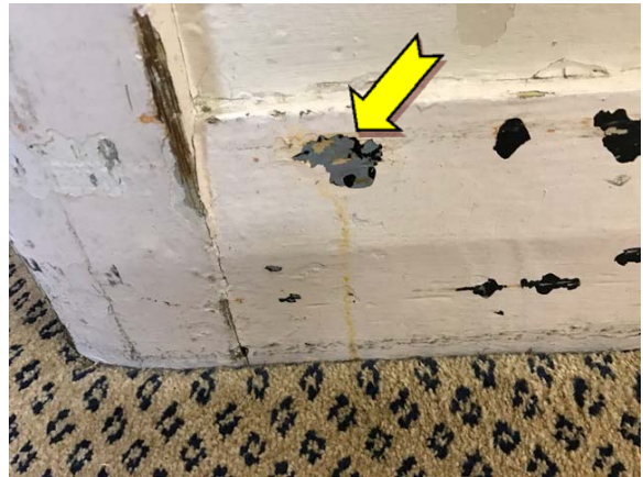
Photo 4. Interior, ground level, southern corridor, skirting boards - suspected lead-containing green upper paint system.
